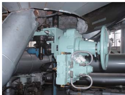
☆Automated reaction tank-bottom valve (special installation)
